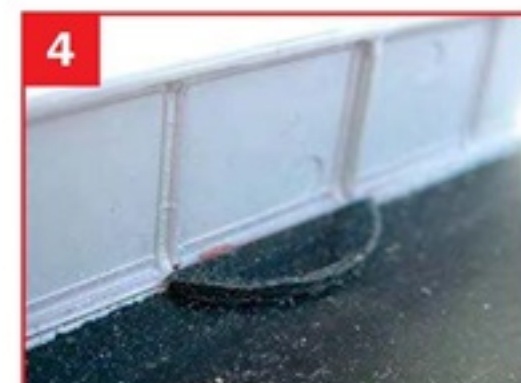
Track guide on bridge deck – Close-up of one of the bridge deck track guides to keep the track centred.
