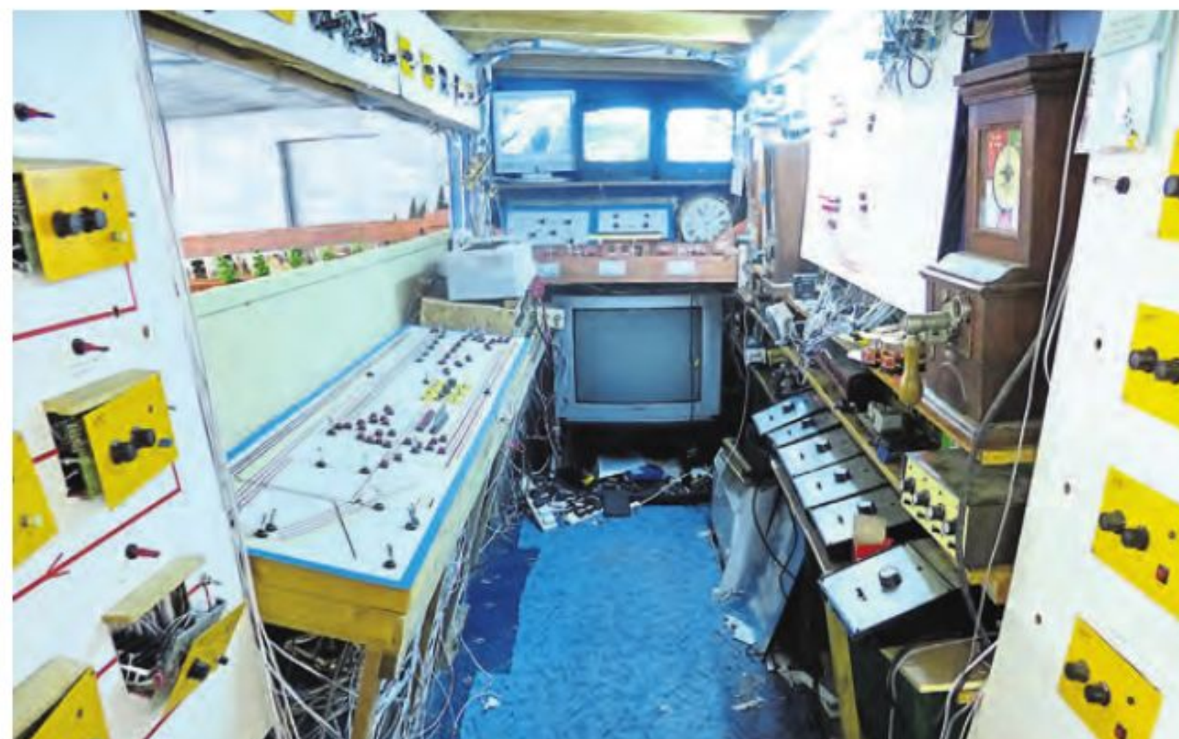
Wires, knobs, switches, diagrams and TV link apparatus are crammed inside the central control room from which the entire layout is operated.
