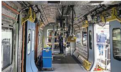
Left: The complex wiring being fitted into a trailer car at Krefeld Works.
