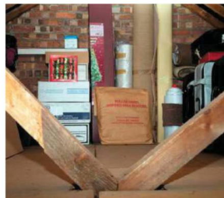
Below: Check that the floor joists are strong enough to support a layout - and humans. Always seek expert advice before making any structural modifications. NICK LYLAK/ALAMY
