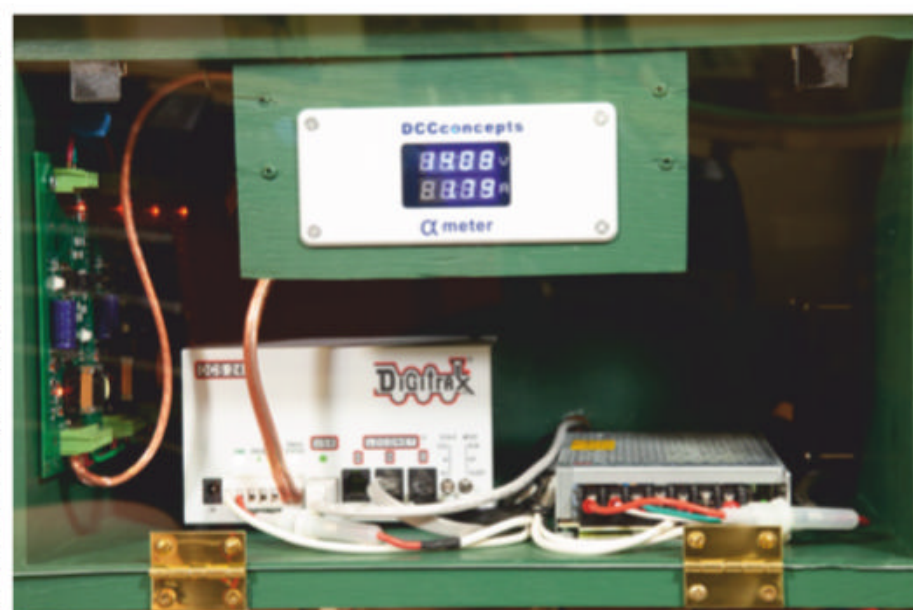
3 Monitoring power. Larry installed his Alpha Meter in a box mounted under his layout fascia along with his Digitrax DCS240 command station, power supply, and DCC Specialties PSX-4 power manager. The 65 locomotives on Larry's layout are only pulling 1.79 amps while at idle.
