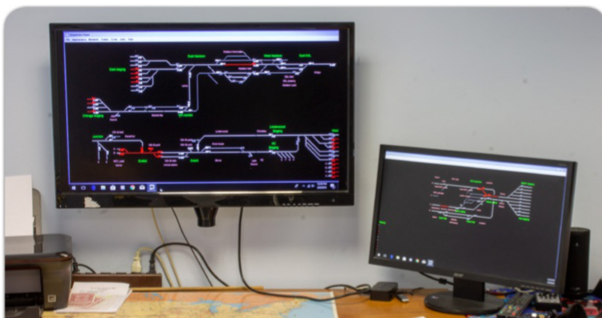
The dispatcher's desk features modern Centralized Traffic Control screens that show train locations and signal aspects.
