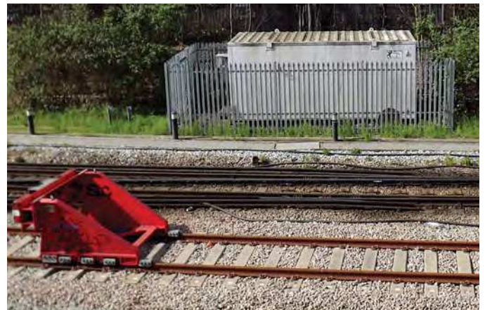
Relocatable Equipment Buildings (REB) house vital signalling equipment for an area, such as this example at West Croydon.
