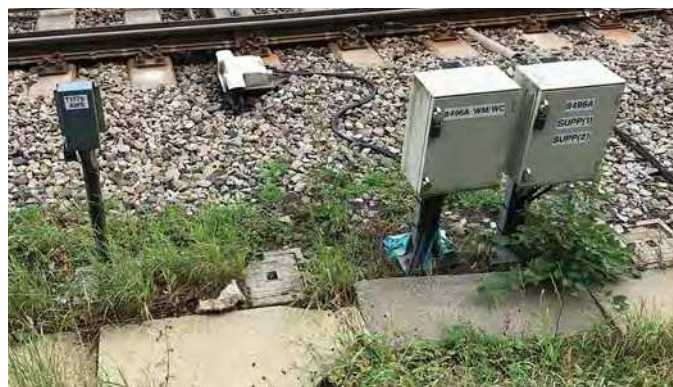
A variety of Disconnection Boxes at Tilehurst. On the left is the Dis Box for an AWS magnet, whilst on the right are boxes for a point motor (left) and supplementary detector (right). The supplementary detector can be seen between the two types of box.
