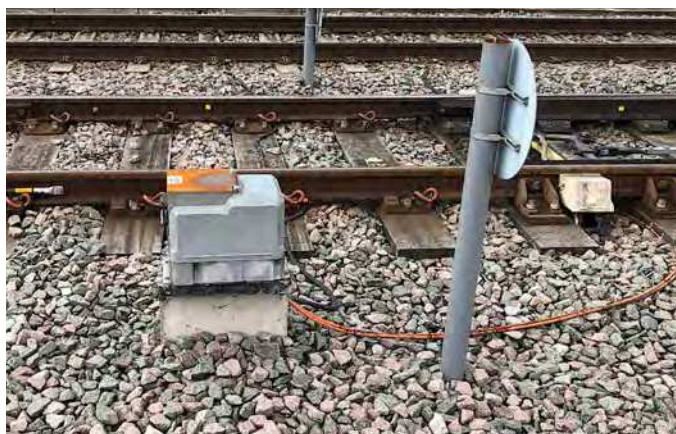
Clamp lock hydraulic motors are the preferred point motor on the modern railway. This is a clamp lock power pack within Reading Train Care Depot.
