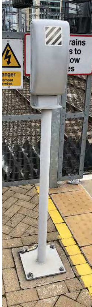
Lineside telephone points enable staff to contact the signalling team. This platform-mounted signal post telephone (SPT) is located at Reading station.
