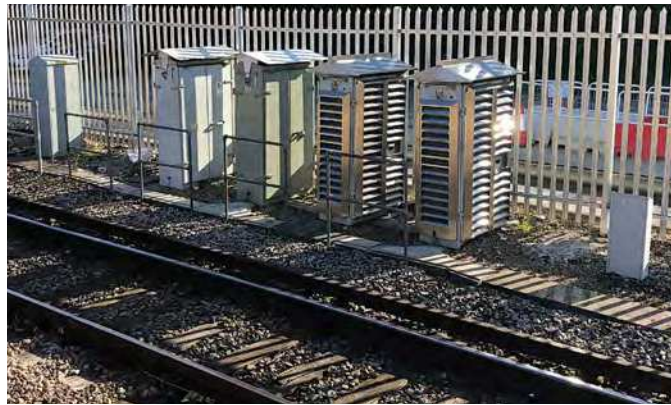
Signalling location cases appear in a variety of guises, such as these at Guildford railway station.
