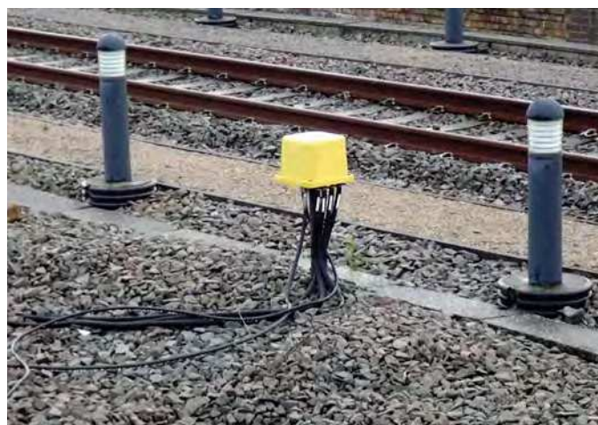
Axle counters are gradually replacing traditional track circuits as the preferred form of train detection. This is a Thales EAK30H electrical junction box for an axle counter head at Milton Keynes.
