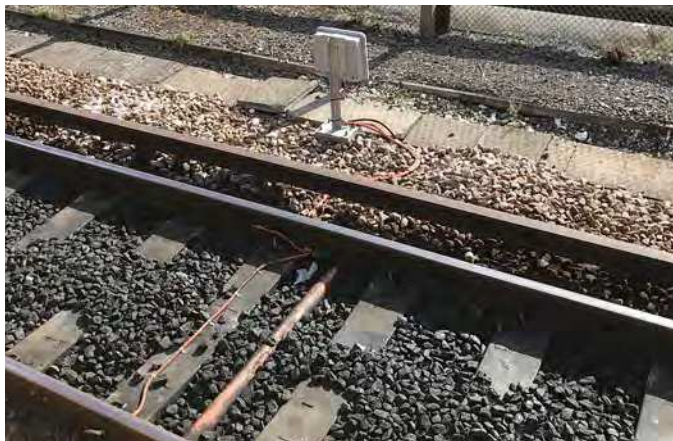
A TI-21 audio frequency track circuit tuning unit alongside platform eight at Guildford railway station.
