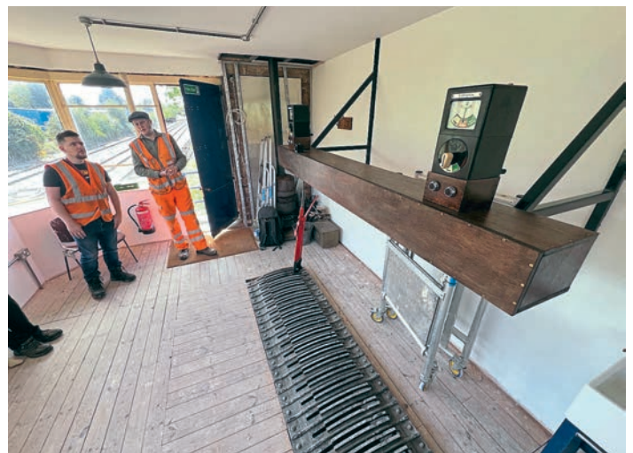
The new block shelf installed inside Hotchley Hill signalbox. TOM INGALL/GCR(N)
