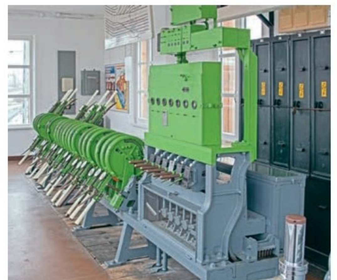
A very different set of levers inside the display signalbox alongside the main line.
