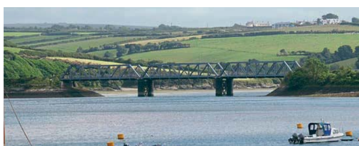
The three-span LSWR girder bridge which crosses Little Petherick Creek, near Padstow. The spans are formed of two Pratt trusses, nine cross girders and three wind braces, giving a deck width of 16ft 3in. It was built by Derby contractor Eastwood Swingler & Co. The ironwork was brought by rail to Wadebridge before being carried on barges down the River Camel to the construction site. ROBIN JONES
