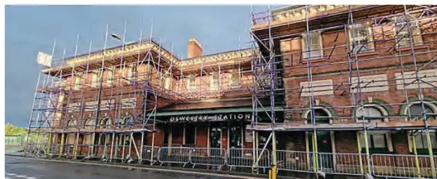
The Cambrian Railways headquarters building and station in Oswestry await essential repairs. SHROPSHIRE COUNCIL
