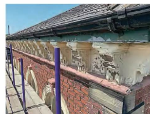
Damaged corbels on the building, along with guttering, soffits and drainpipes, will be repaired and repainted. SHROPSHIRE COUNCIL
