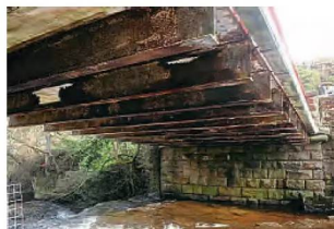
The deteriorating girders beneath Bridge 27A, which provides access to Goathland station. MIKE BRAHAM/NYMR
