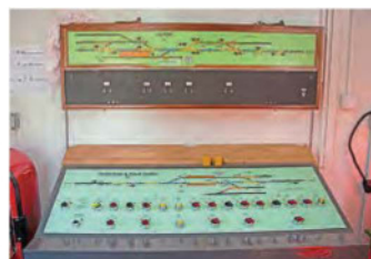
The control panel for the new 'box at Medstead & Four Marks station also displays train and signal indicators for the terminus at Alton.
