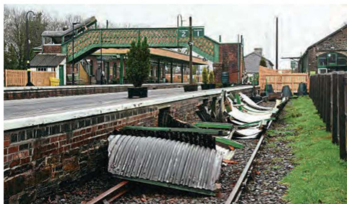
Pictured is the damaged footbridge with (on the right) the larger roof sections saved in the bay platform line. DAVID HUNT
