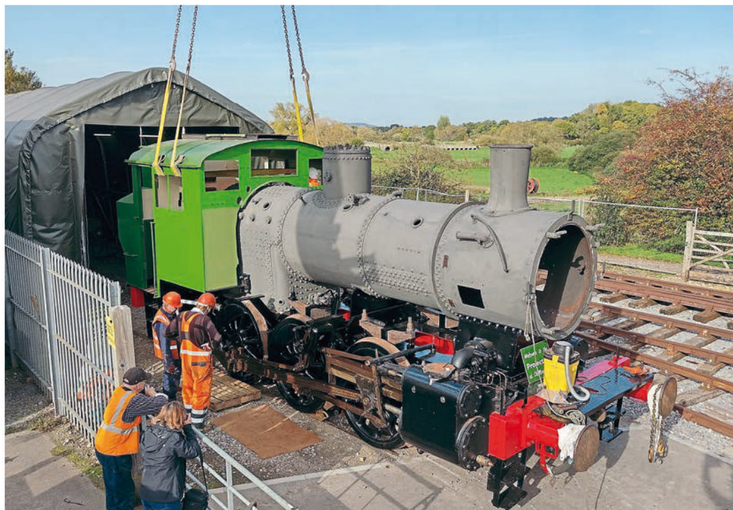
The boiler and cab of Yugoslavian S100 0-6-0T No. 195462-699 (BR 30075) are now back on the frames as the locomotive takes another step towards a return to steam. PROJECT 62
