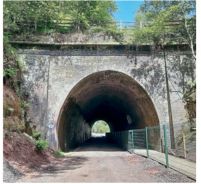
Birchall Tunnel in the sunshine with the track cleared and the concessionary footpath in place. NICOLA FOX
