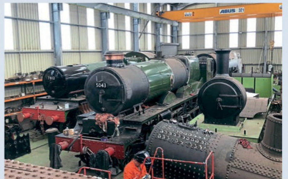
Earl of Mount Edgcumbe's boiler back in the frames at Tyseley. VT
