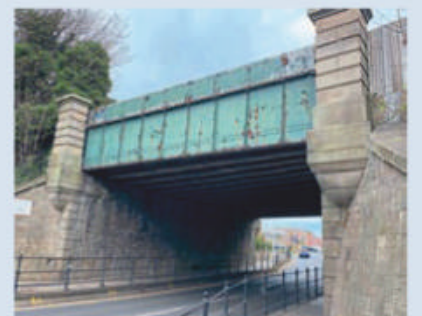
In need of a repaint and getting one sometime soon: Darlington's historic North Road bridge. NETWORK RAIL
