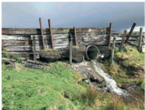
The current condition of the culvert led to it being condemned during a professional track inspection. DVR
