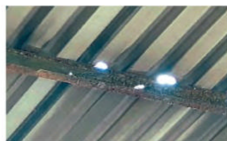
Holes and purlins in the roof of Bridgnorth motive power depot. ANTHONY BARTLAM/SVR
