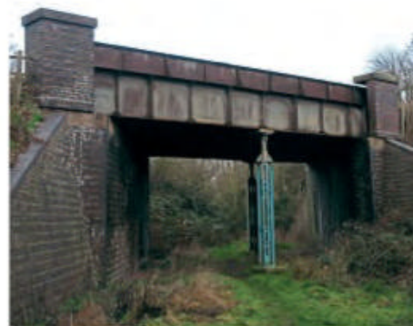
Collin Lane road overbridge, near Willersey on the Broadway-Honeybourne line, is described as being "in a very poor state with brickwork damage and seriously corroded steel". It is propped from beneath in order to carry heavy lorries. JO ROESEN
