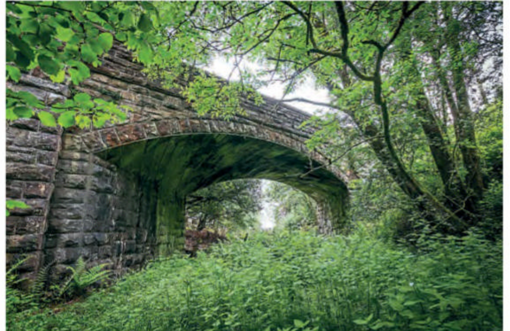
In a major about-turn, Lochanhead bridge on the former Stranraer to Dumfries line will now be repaired rather than infilled. HRE GROUP
