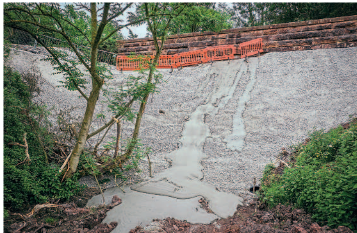
Great Musgrave Bridge infilled by concrete, despite protests. THE HRE GROUP
