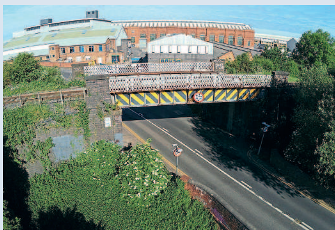
Bridge 326, which takes the Great Central Railway (Nottingham) over the busy A60 at Loughborough, needs major refurbishment – possibly a new span structure – before it can carry trains again. EMRT
