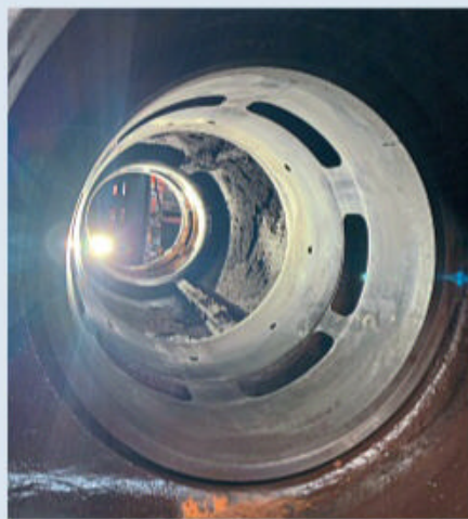
The driver's side piston valve chest showing the deep wear between the ports. SIMON HUNTER
