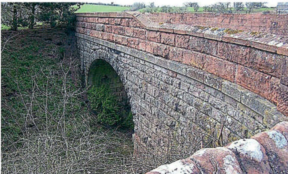
Bridge No. 25 on the trackbed of the NER's Eden Valley route in Cumbria which, if lost would prevent two heritage lines one day linking. MIKE THOMPSON
