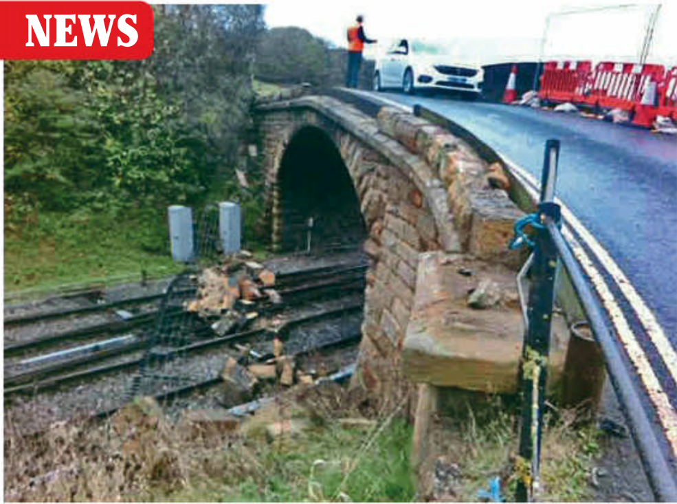
Track obstruction: Debris lies on the track of the North Yorkshire Moors Railway on October 20, shortly after the bridge parapet above had been hit by a lorry. The incident caused the cancellation of the railway's flagship 'Optimist' nonstop service from Pickering to Whitby. NORTH YORKSHIRE COUNTY COUNCIL
