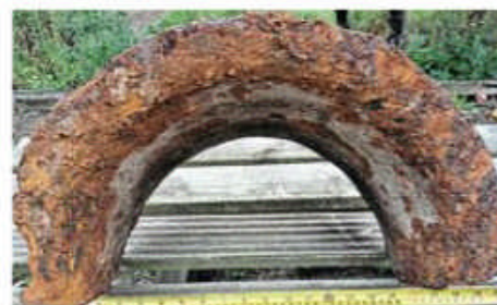
The rusting firehole deflector plate which was uncovered at County School. MNR
