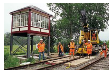
The former Oddingley Crossing signal in position at Shottle. EVR
