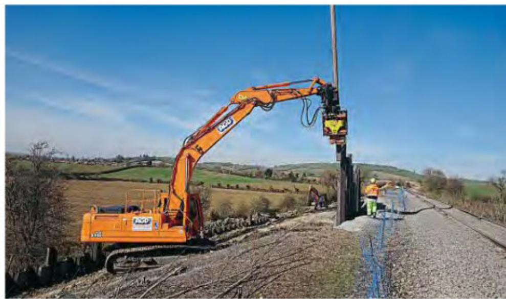
Work on the landslip, seen underway on March 23, has now been halted because of the coronavirus pandemic. JONATHAN TAYLOR/G/WR
