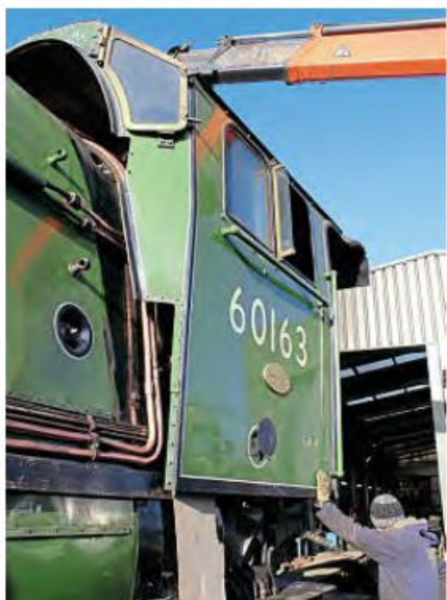
Above: Following its routine winter maintenance, the cab of Tornado is seen being lowered back into place at Leeming Bar on February 26. ATSLT.
