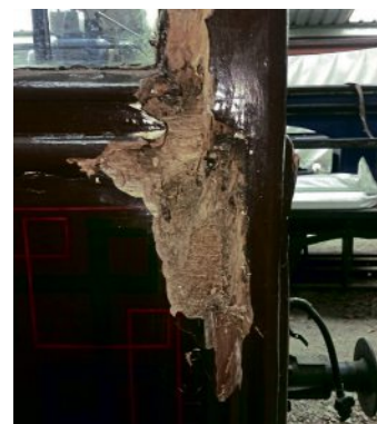
A close-up of one of the east-end corner pillars, both of which need to be replaced. TOM CURTIS/ TR
