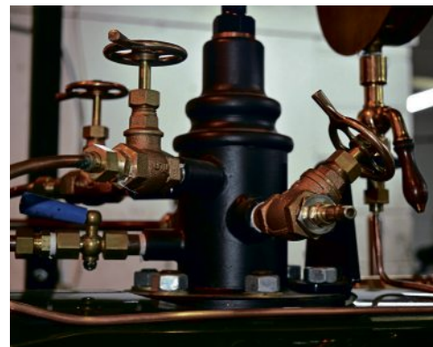
This is a close-up of the steam manifold showing the feed to the pressure gauge (bottom); the blower pipe (centre left foreground) and behind, the steam feed to the drain cock mechanism. The disconnected take-off is the steam feed to the injector, temporarily in use as the compressed air intake for testing purposes.
