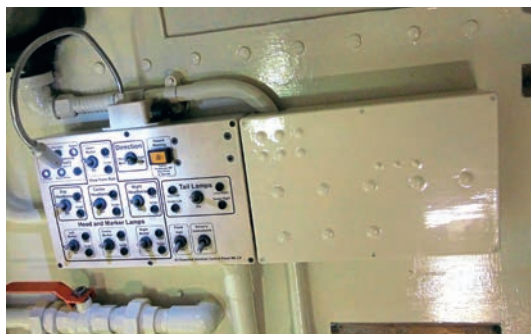
The essential services control panel fitted to Tornado . An improved version of Tornado 's proven electrical systems will be fitted to P2 No. 2007 Prince of Wales . ROB MORLAND
