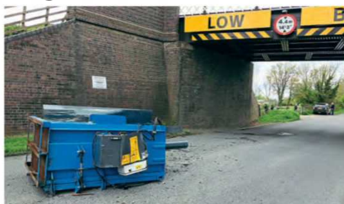
The lorry's load lies in Station Road after the May 1 bridge strike. The incident caused only minor damage but it was spectacular in that the ill-secured load was swept straight off the truck. G/WR
