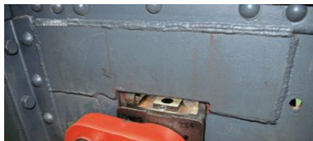
Further evidence of the hard working life experienced by Liassic at Southam is evident in this view of a welded repair carried out on the portion of the right-hand mainframe immediately above the horn area. This part of a locomotive's mainframes is particularly vulnerable to the stresses encountered during normal working.
