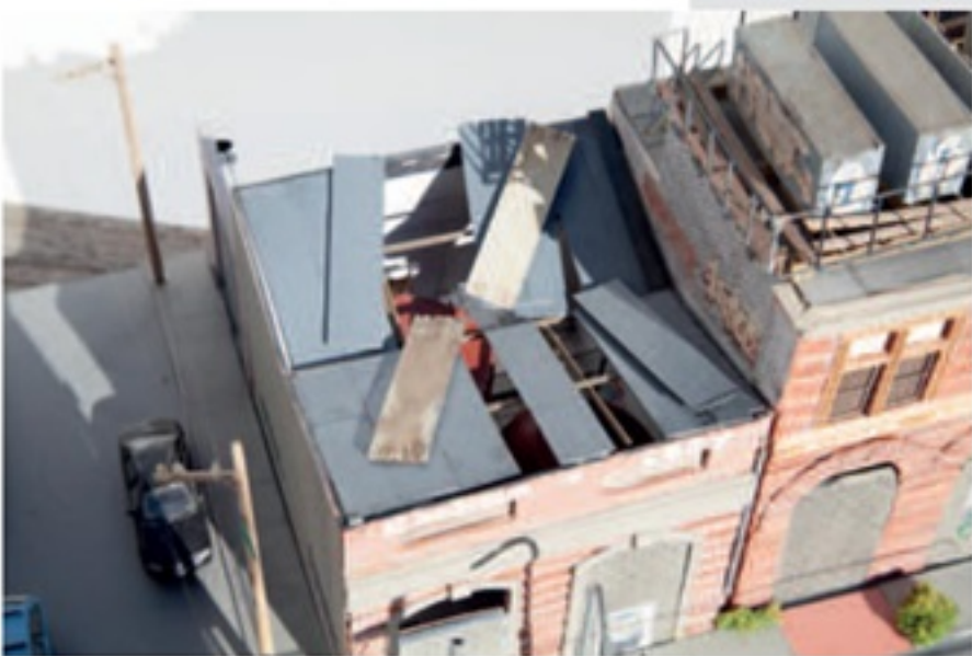
Above The deteriorating roof reveals part of the interior.
