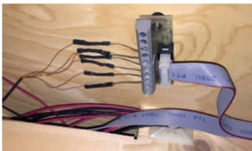
Right The screw terminal to ribbon cable adaptor under a signal – the fine individual feeds are soldered to heavier wire within the black shrink wrap.
