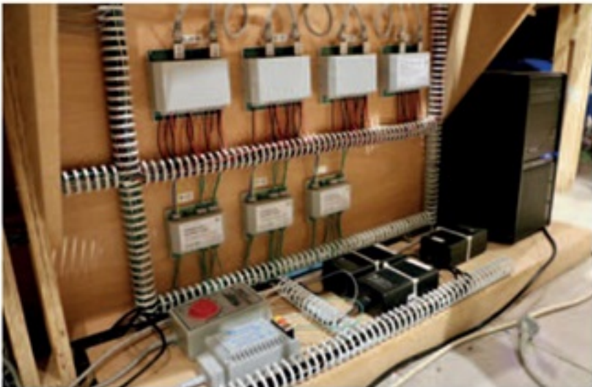
Above Filisur electrical panel: at the bottom, transformers for the power supplies and boosters. Vertical: feedback modules above and decoders for the point motors below.
