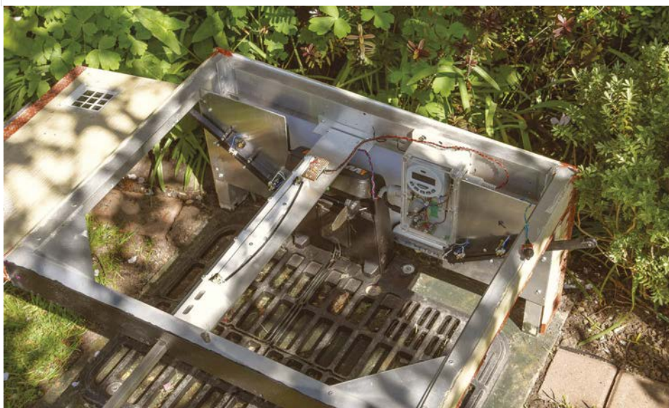
With the top and two doors removed, you can see all three actuators extended and the arrangement of the control box.
