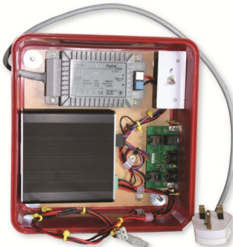
The layout of the equipment in the box.
