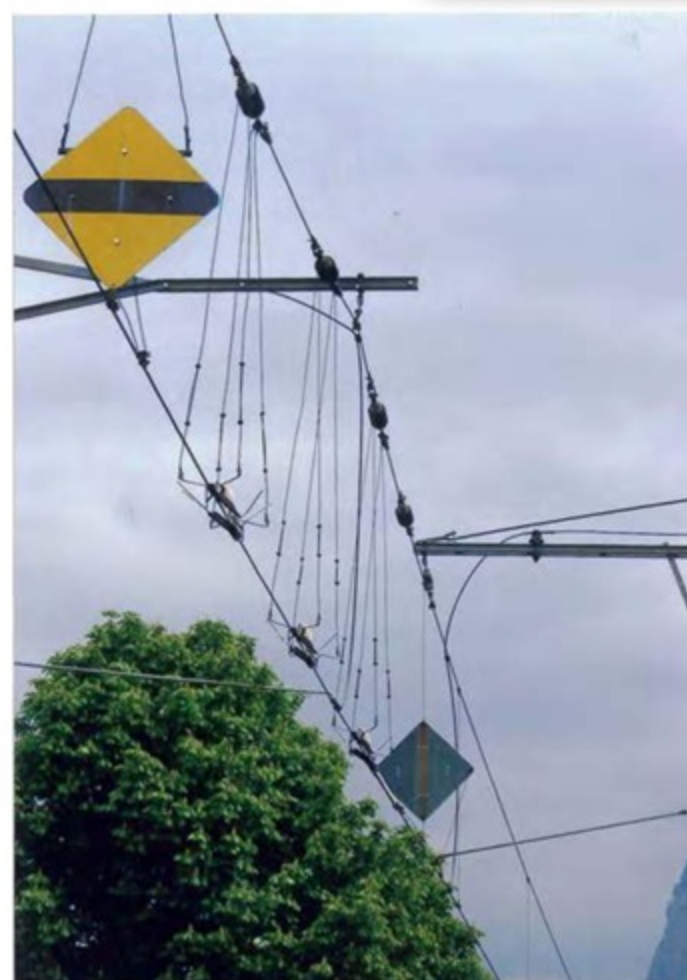
Right The complicated electrical isolation at Meiringen MIB where the 1,200v d.c. meets the ZB 15kV 16.66Hz a.c.
