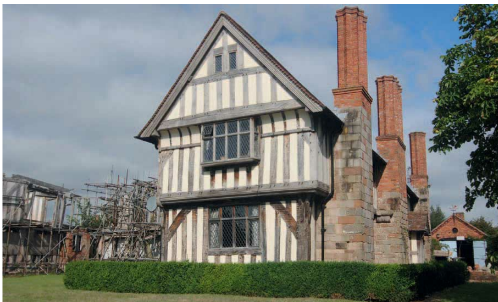
The gable end of the north wing of 'Sinai Park House'. Note the scaffolding holding up the crumbling skeleton timber frame. This part of the building, as
