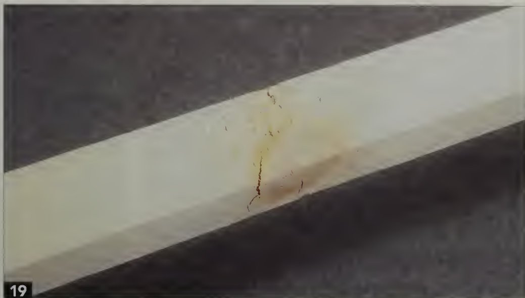
19 Avoid boards like this 1 x 2, which has a knot that severely compromises its strength.
