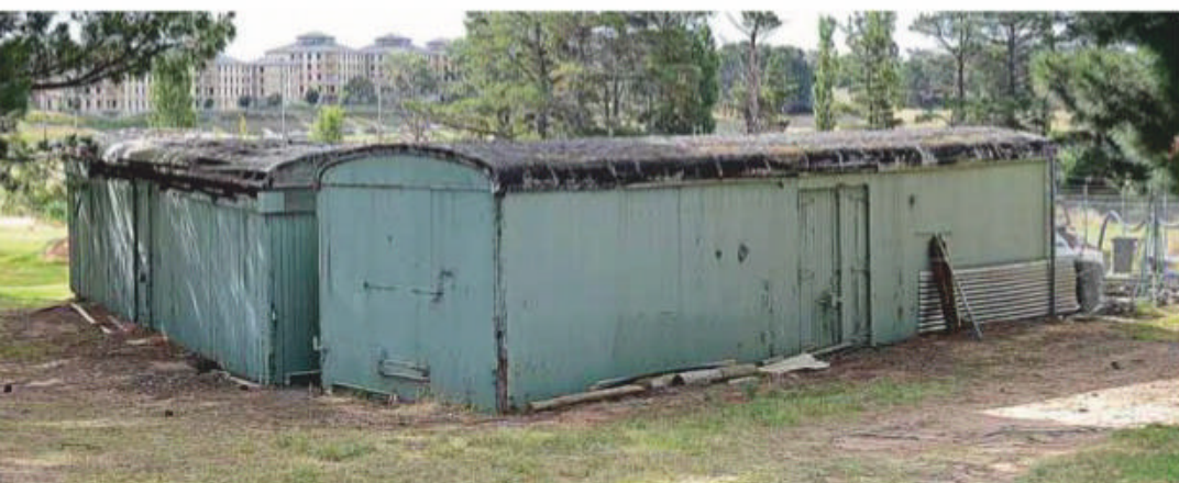
The other side of the vans shows much potential for the superdetailer with the deteriorating roof, particularly on the left-hand van, and other details such as the corrugated iron covering damage to the side panel and the many 'bits and pieces' lying around.
