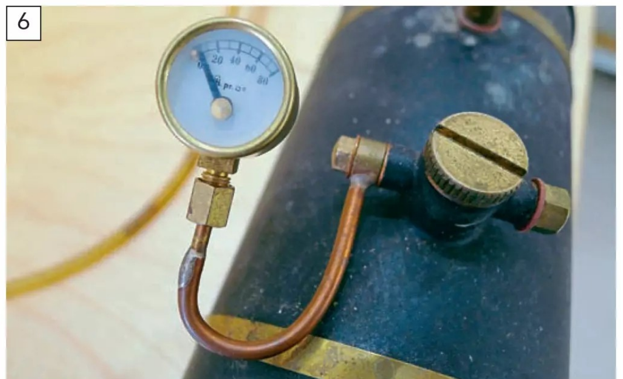
The pressure gauge looked to be in good condition, although there was no red line at the working pressure as required by the Boiler Test Code, 2018.
