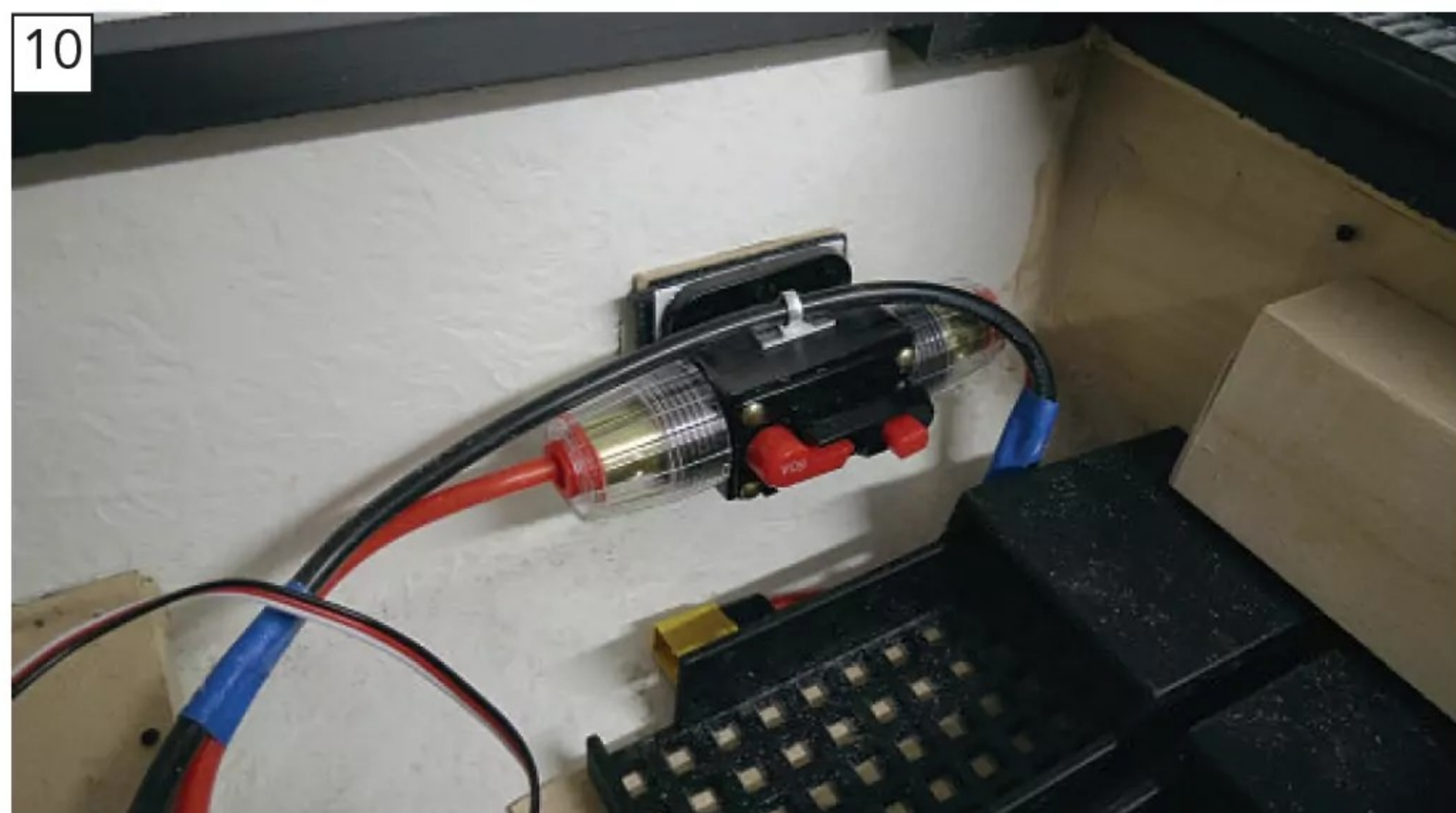
The breaker switch harness protecting the ESC.
