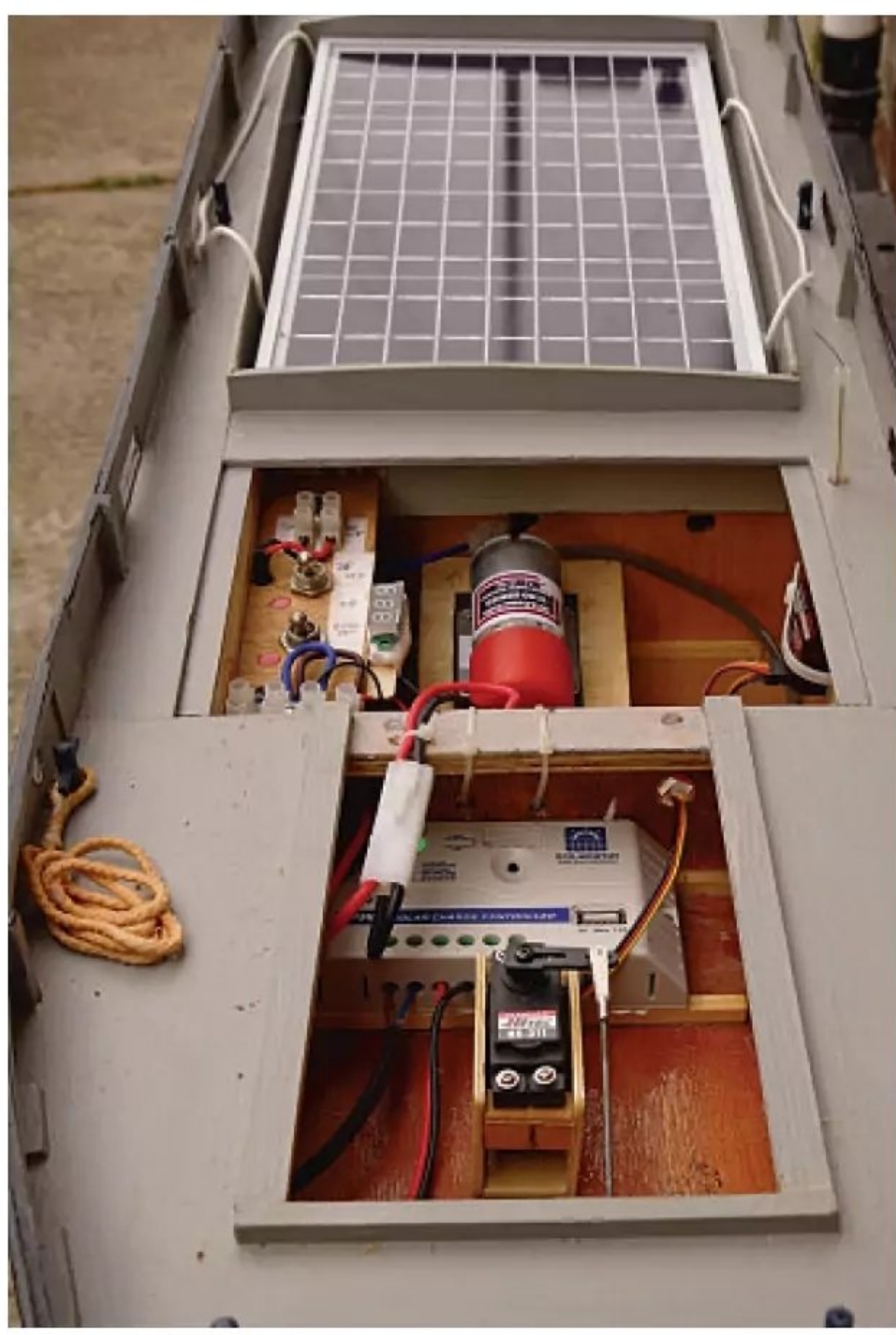
The final layout of electrical equipment: the solar panel sits on four wooden dowel pegs above the battery. The white cord/rope forms handles, which allow the solar panel to be lifted out to gain battery access.
