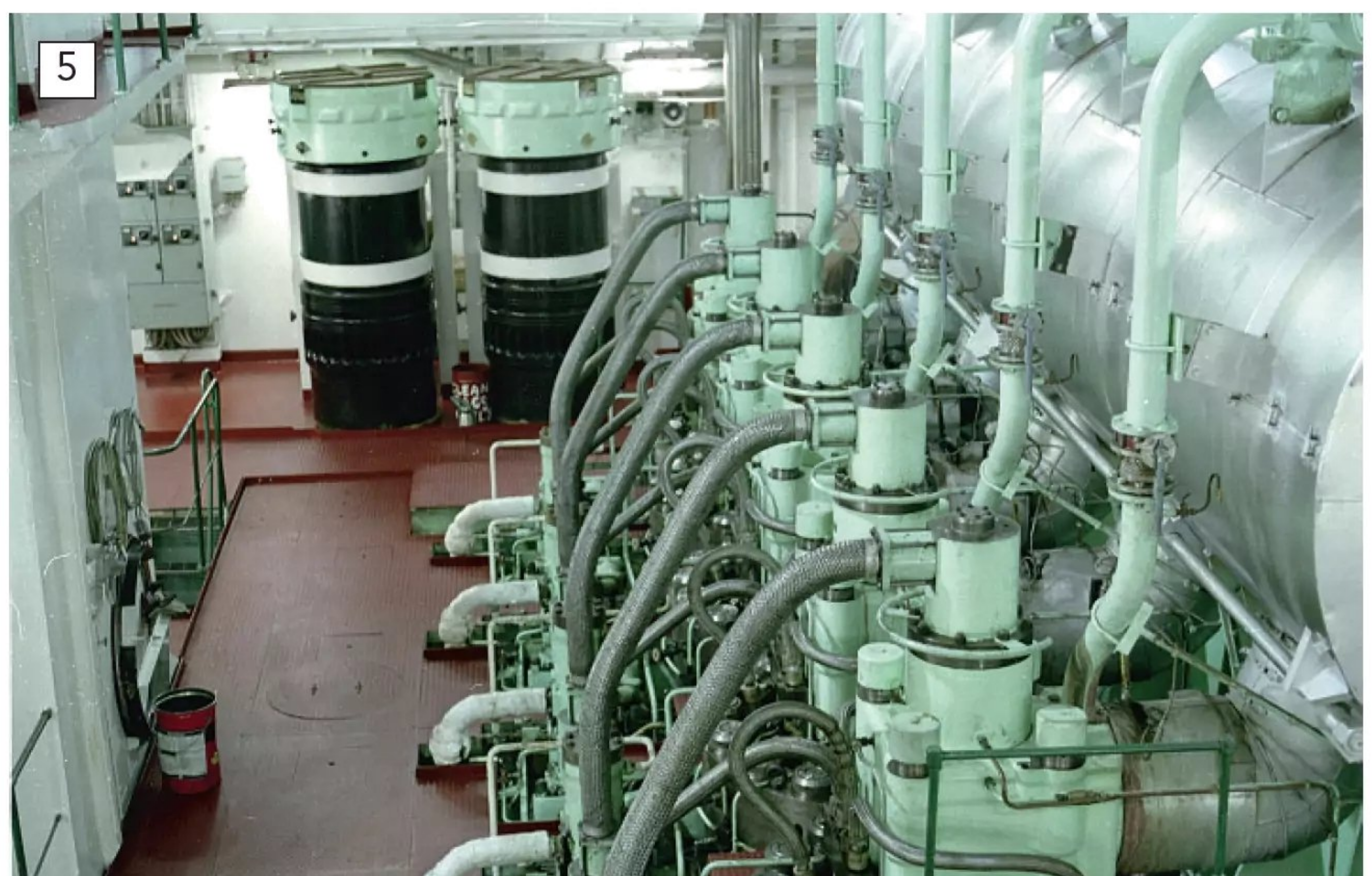
A traditional cargo ship could have the main diesel engine crankshaft connected directly to the propeller shaft. Again, significant damage would be caused if longitudinal forces were to be applied to the engine crankshaft. This slow speed diesel is directly connected.
