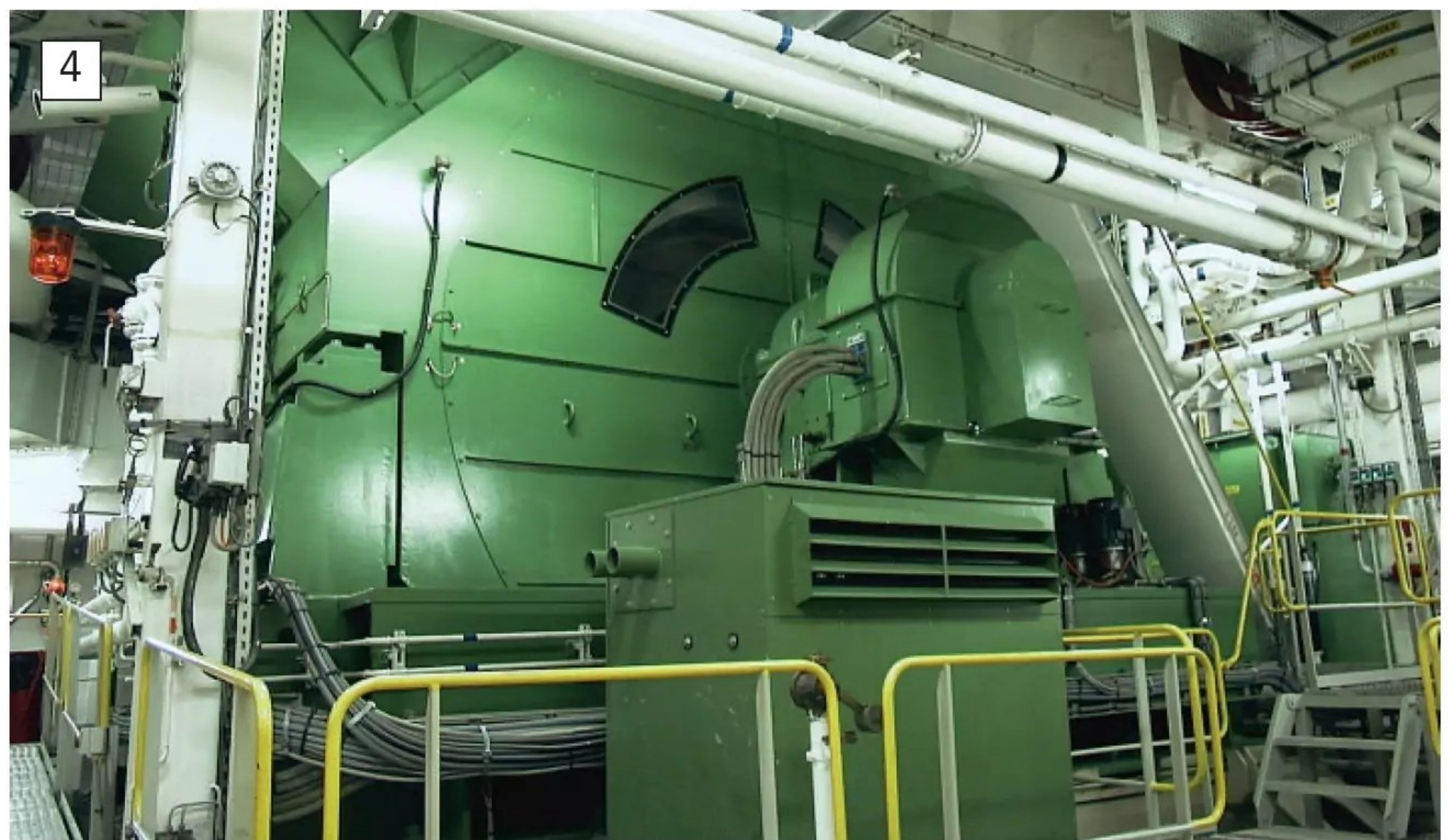
As with any electric powered model boat, a diesel electric ship has an electric motor connected directly to the propeller shaft. The rotor of this motor must be isolated from the thrust forces to prevent damage, or at least undue wear.
