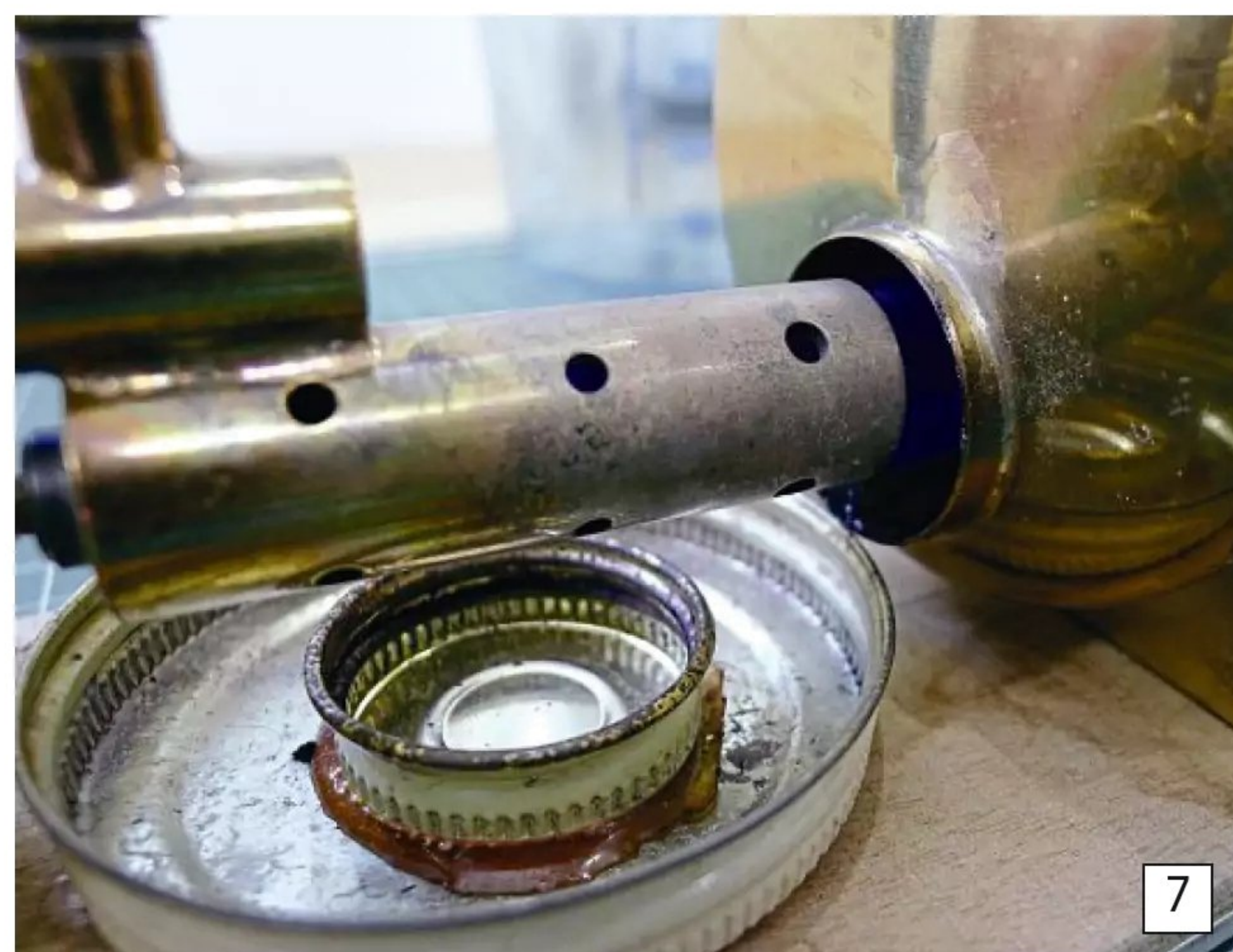
Once everything is settled down and established, you should see and hear a nice clean blue flame at the boiler and feel the hot exhaust gasses at the top of the flue.
