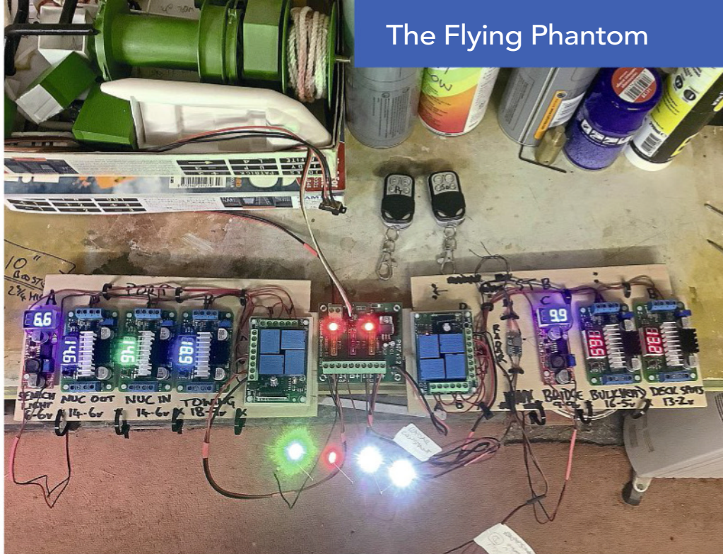
The heart of the lighting system, also showing the two fobs that control the relays.
