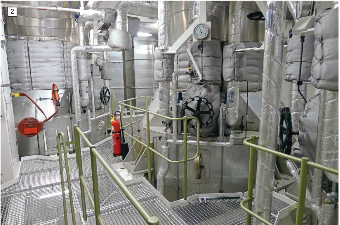
Even nowadays steam pipes will either be wrapped with thick insulating cord covered in foil or, in this case, thick insulating material with the foil covering pre-applied.
