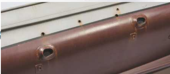
BELOW: Rafal has also incorporated leaks around the spill holes and vines in selected areas.
