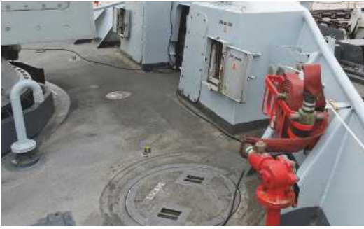
LEFT: Moving inboard of the breakwater we have a view of the arrangement over to starboard with the rising main for firefighting in the foreground.
