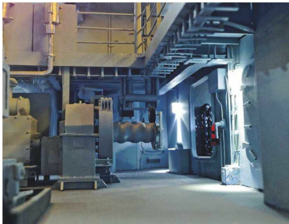
BELOW: Looking into the LED illuminated winch working area.
