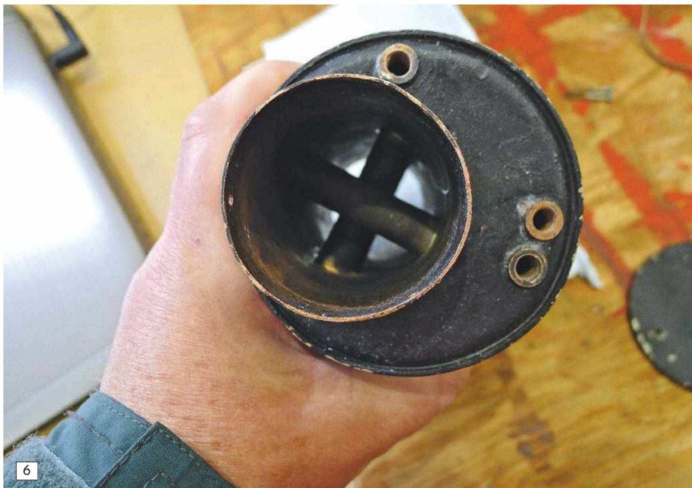
Photo 6. Cross tubes inside the flue indicate a potent boiler, but these need inspecting thoroughly both from the outside and as much as possible, from the inside as well.
