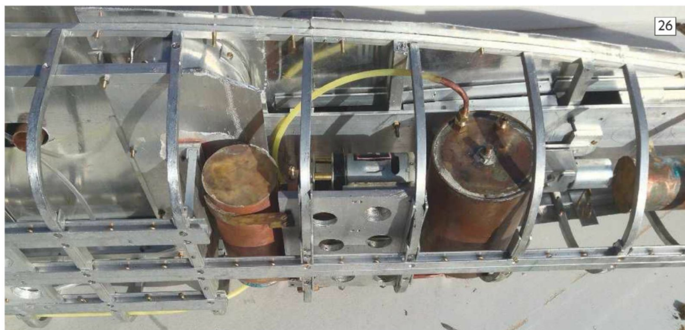
Photo 26. Close-up of the fuel and water tanks with the pump drive motor between them.
